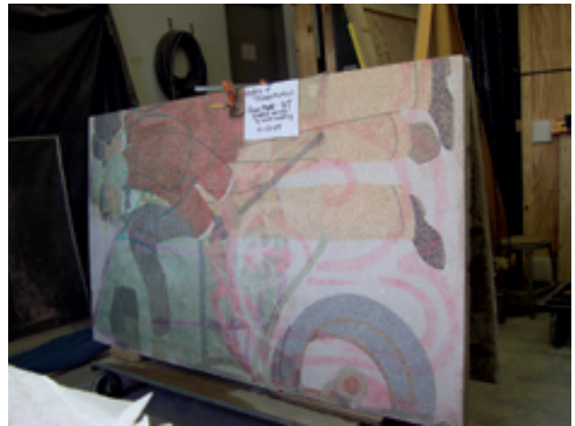
Fig. 5 Panel #25, showing insoluble graffiti ghosting that required removal by powder blasting, and texture of petrachrome.
