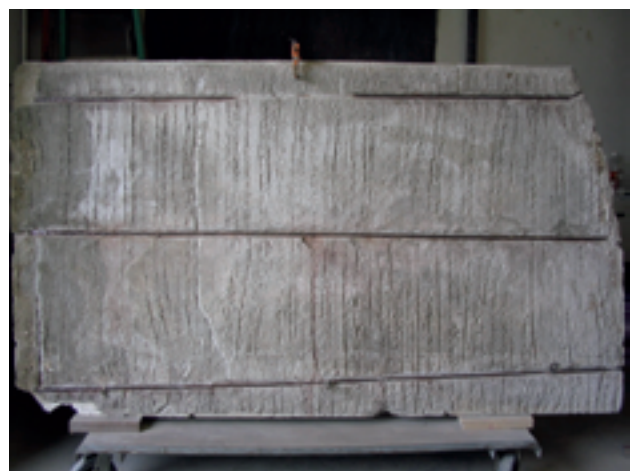
Fig. 6 Panel #59, showing exposed rebar supports before treatment.
